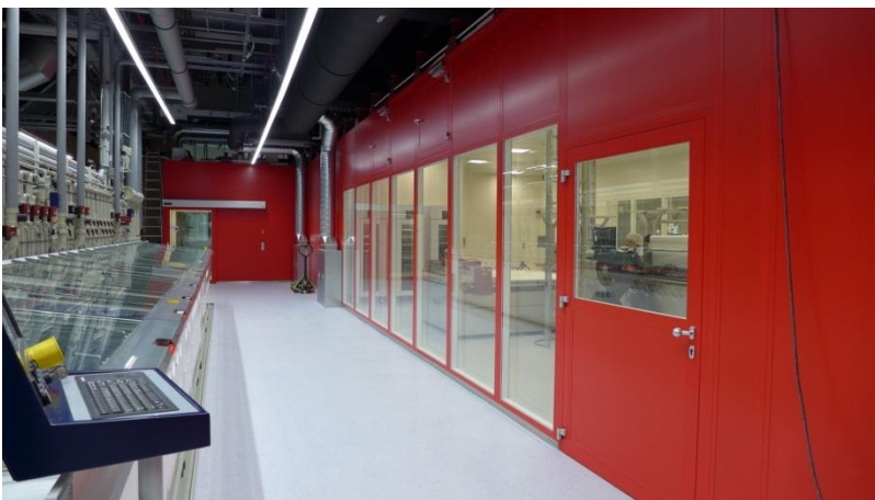
Photo: During reconstruction, production was expanded to include cleanrooms (ISO Class 4 and 5).
