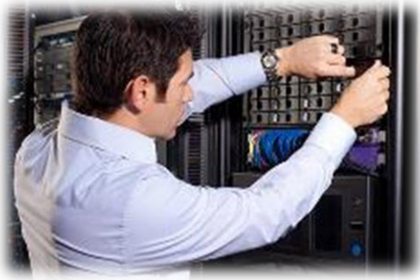
Data Center: rack mounted power supply...
