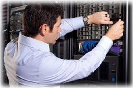
Data Center: rack mounted power supply...
