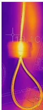
Figure 4: TBL over-current test at ambient temperature of 19.1°C
